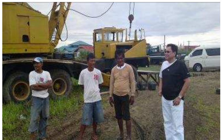
HANDS-ON VISIONARY. Engr. Dingo Bonifacio, the brain behind Project Masantolenos inspects the site and gives instruction to the workers.
